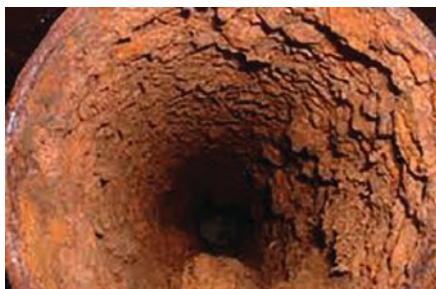
Even the most corrosion resistant metals are still susceptible to galvanic and electrolytic corrosion, resulting in scale build-up, which reduces flow rates and increases pressure drop.
