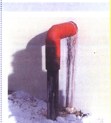
Figure 1: PVDF pipe failure due to presence of sulfur trioxide.
