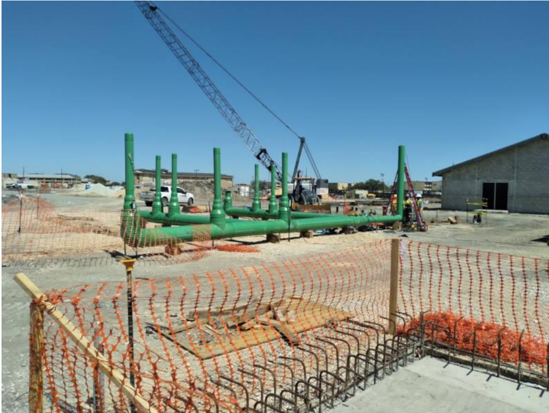
The Air Force's new basic training facility required large diameter pipe and fittings to move 155°F (68°C) water effectively throughout the campus at 90 psi. Using PP-RCT pipe also enabled sections of the system to be fabricated and lifted into the trench. Courtesy: Asahi/America
