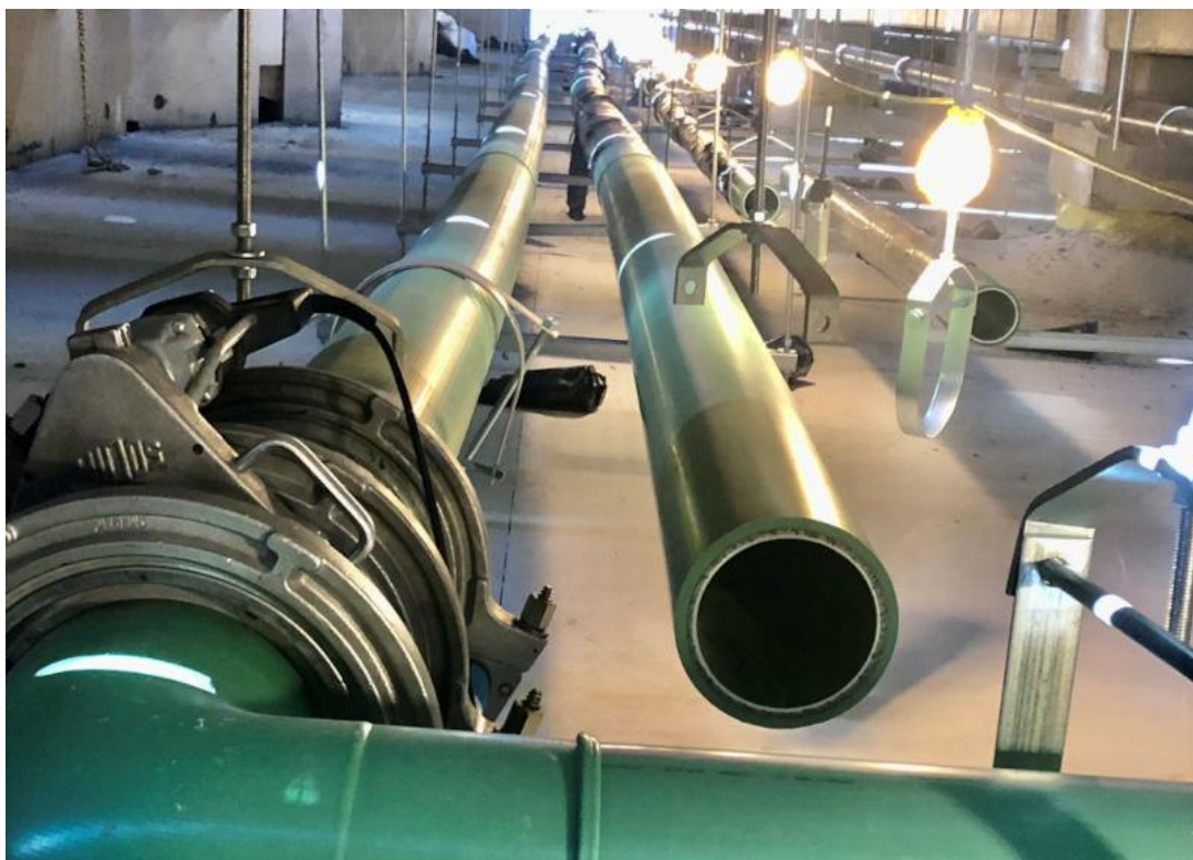
Long runs of PP-RCT pipe are in tight crawl spaces below the first floor. Because of the polypropylene pipe's light weight there was no need to use heavy duty hangers or supports. Courtesy: Asahi/America
