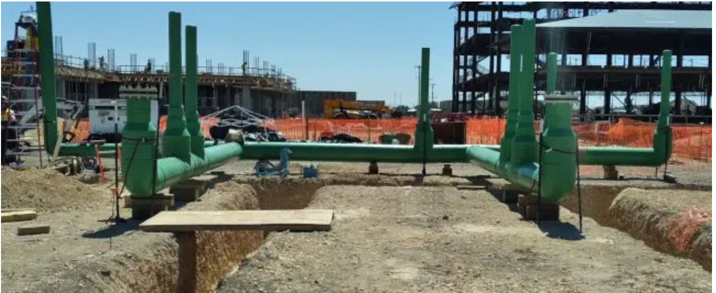
The Air Force's new basic training facility required large diameter pipe and fittings to move 155°F (68°C) water effectively throughout the campus at 90 psi. Using PP-RCT pipe also enabled sections of the system to be fabricated and lifted into the trench. Courtesy: Asahi/America
